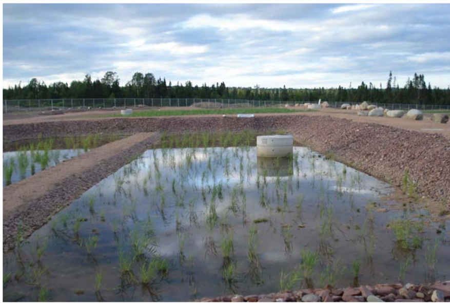
Figure 1. Stormwater bed during commissioning.
