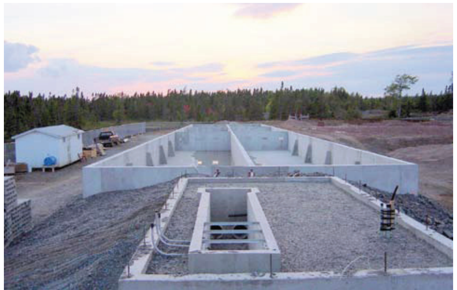
FIGURE 1. View of grinder building foundation with pit for grinder and spiral lift; the settling chambers are directly behind.
